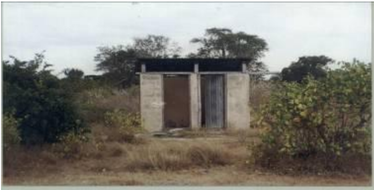
Toilets construction- one way of improving sanitation in schools and watering points
